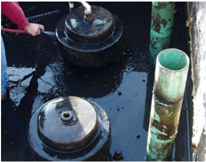
Failed alternating bell siphons to be replaced with Flouts
